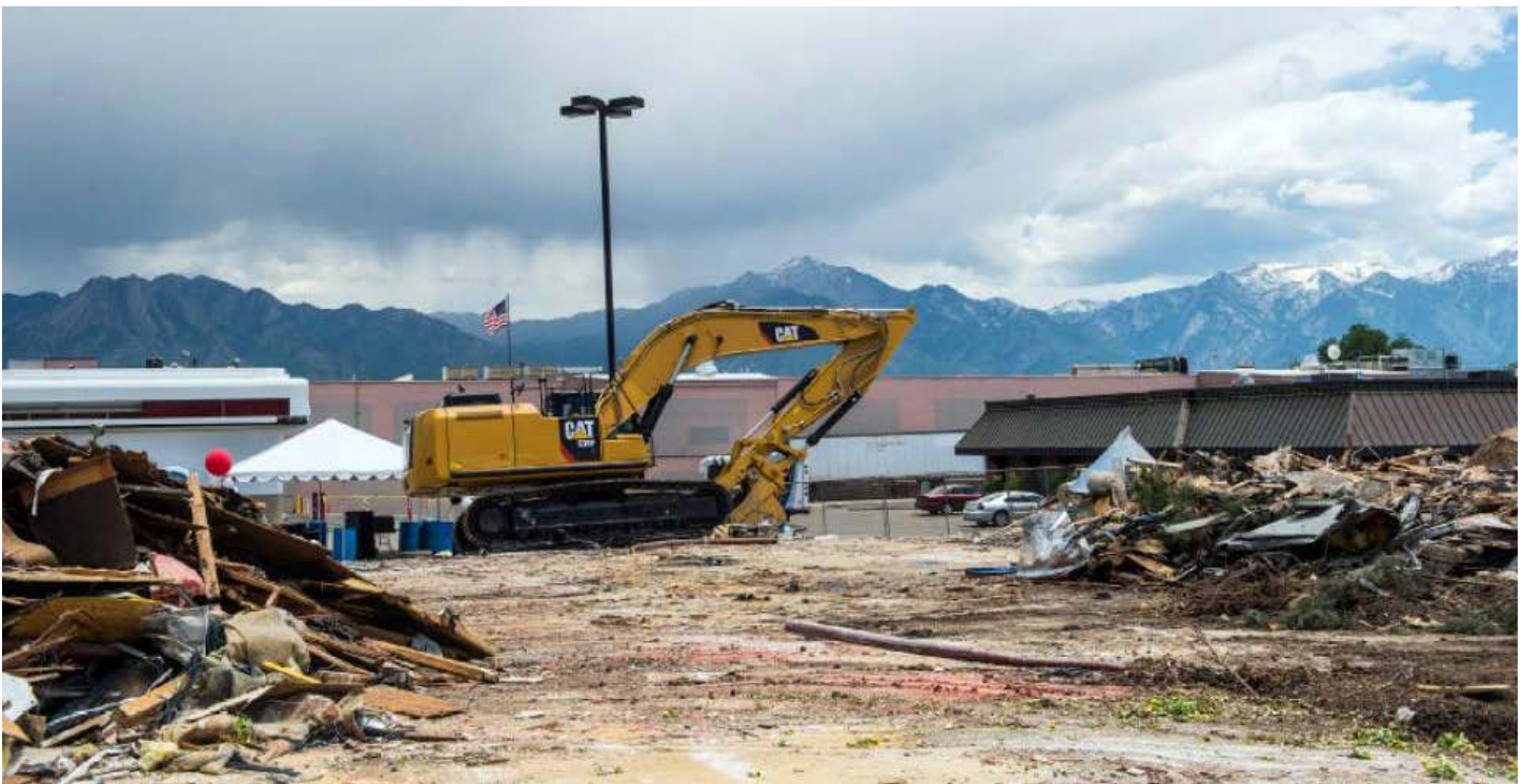
(Chris Detrick | The Salt Lake Tribune) Demolition of vacant businesses near 5400 South and 1750 West Tuesday June 9, 2015.
